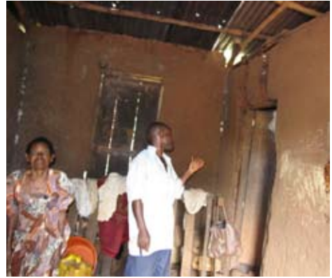
Theresa and her son inside their former house; note the dangerous cracks in the walls and the holes in the iron sheets that leak during rain causing coldness which affected the old woman's health.
