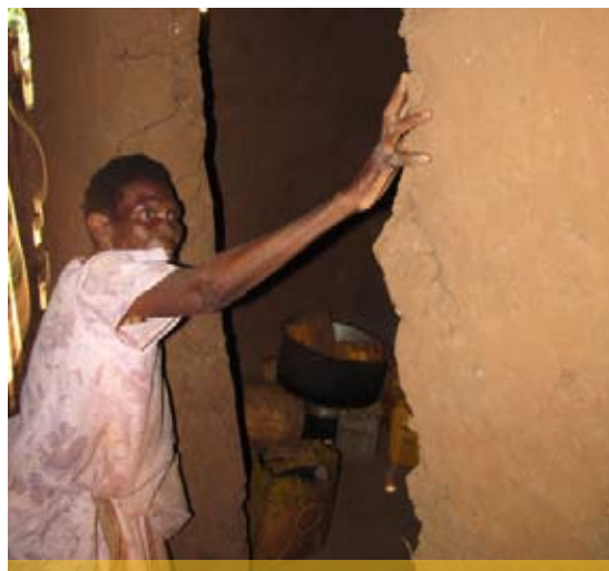
Grandmother Gladys showing the damaged wall which caused her household members to vacate the entire section of the house to use the sitting and dining room.
