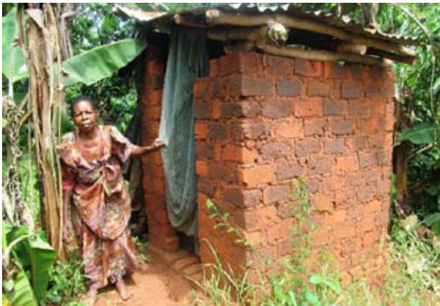
Theresa near her unsafe old latrine; note the cloth that was used for a door which leaves no room for privacy
