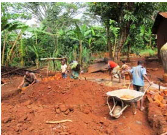
House construction at Gladys's place; all household members actively participating in the construction process.
