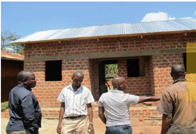
Board Vice Chairperson, Accountant and the Finance and Administration interacting with engineer at the construction site of Jjaja Gladys's home.
