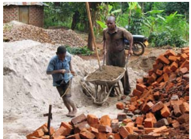
Joylance's grandson helping the engineer to carry sand to the construction site.
